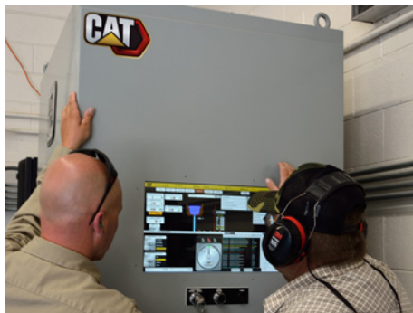
The new switchgear provides remote visibility to ensure better protection through the newest technology.
