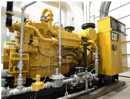
The CHP genset produces about 150 kW of electricity, with 70 to 80 kW used to power the bioenergy facility's water treatment process.
