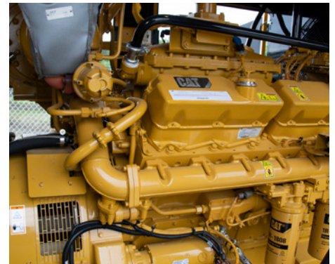
The solar farm is connected to a microgrid that includes energy storage, a Cat® G3412 gas-fueled generator set, and a control system
