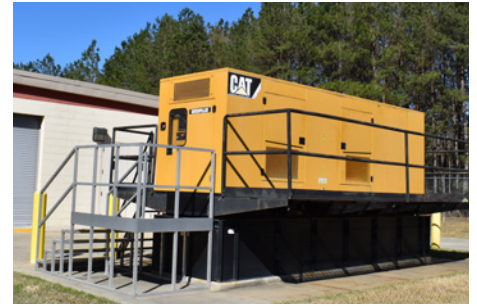
The multitude of Cat generators at Coushatta is necessary to keep various parts of the resort running, from slot machines to hotel laundry operations.
