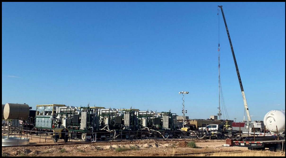
Figure 5: Three GTUIT processing systems on a Permian frac site
