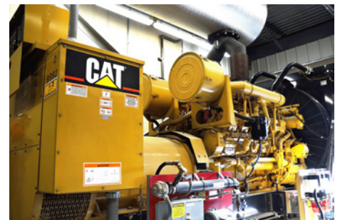
The upgrade at KCI included the control panels on the generator sets, as well as the PLCs, relays and HMI software on the switchgear.
