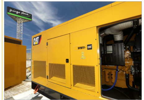
Two DE850E0 power density units were installed at the Pingo Doce grocery store in the city of Póvoa do Varzim.
