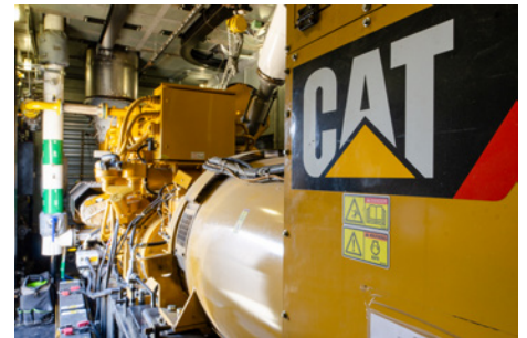
By running its CHP plant continuously, Saint Peter's saves $200,000 to $300,000 per year in energy costs.
