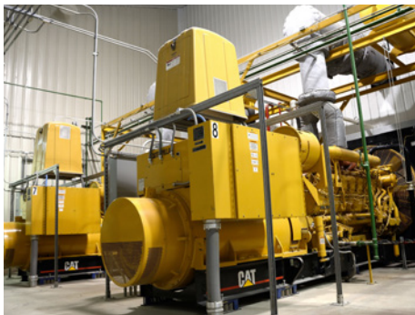
Twelve Cat® 3516B diesel generator sets housed in a stand-alone building next to the main office can economically produce 24 megawatts should the entire city of 8,700 residents lose power.
