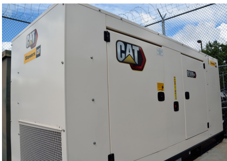
The Cat® D300 GC diesel generator set fits within the footprint of the previous generator set and utilizes diesel fuel tanks already installed at the jail.
