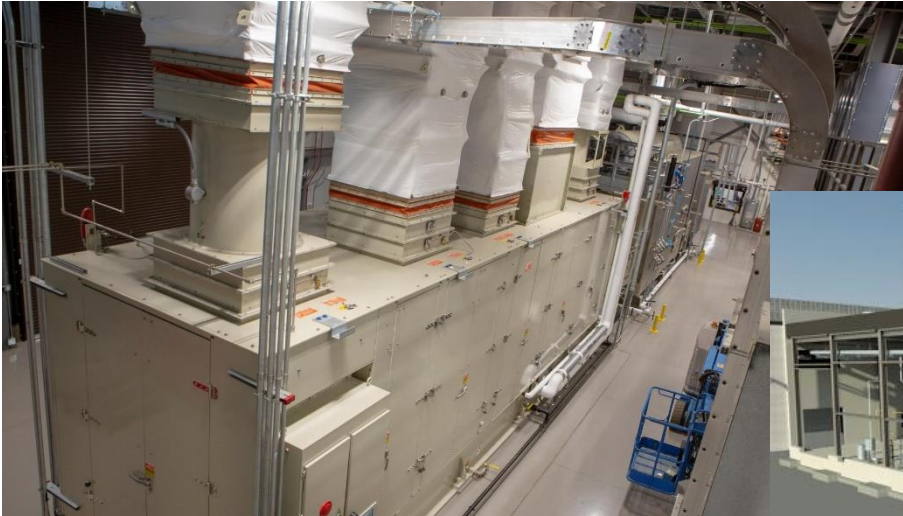
The 7.5 MW Combustion Turbine Prime Mover
