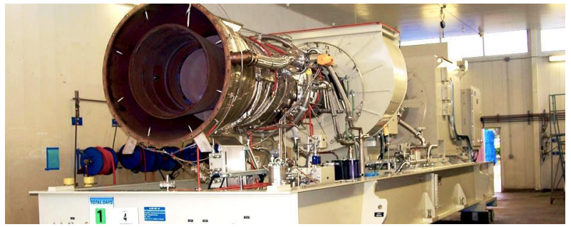
Taurus 70 Combustion Turbine/Generator with Heat Recovery
