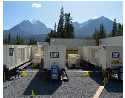
The turnkey solution provided by Finning included the engineering and design, as well as operating and maintaining the plant for the duration of the project.
