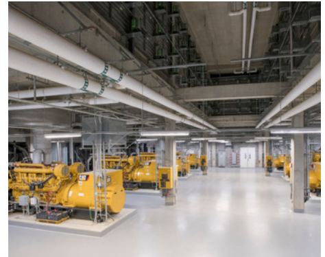
The entire Pensacola campus is backed up by 11 Cat® 3516 diesel generator sets that are housed in two separate buildings.
