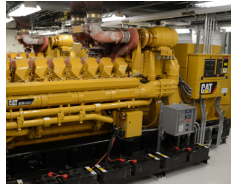
Four Cat® C175-16 generator sets were provided by local Cat dealer Blanchard Power Systems.
