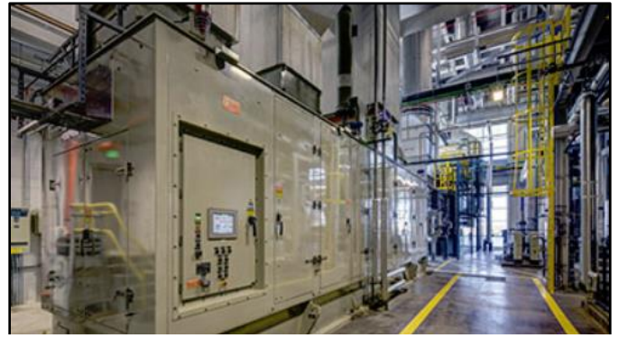
Enclosure for 5.7 MW Solar Taurus Gas Turbine with 50,000 lbs/hour Heat Recovery Steam Generator
