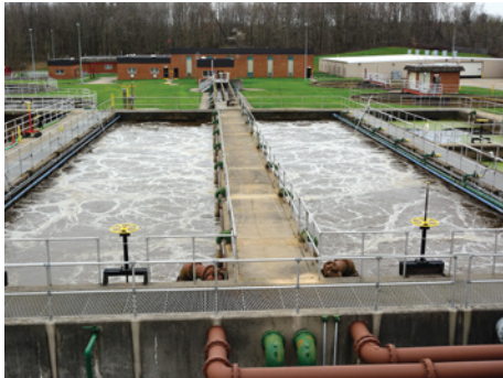
Nestled in a wooded valley about 30 miles south of Cleveland, the Hinckley Wastewater Treatment Plant provides a tranquil setting for ongoing sewage treatment.
