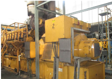
Two Cat® 3612 furnace oil generator sets have been providing power to Din Textile Mills, Ltd. since 1997.
