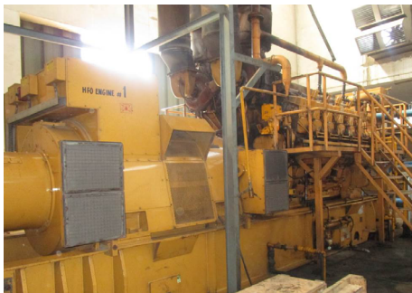
Highly skilled members of Din's technical staff have performed four overhauls on these two generator sets, which have been operating for more than 20 years.
