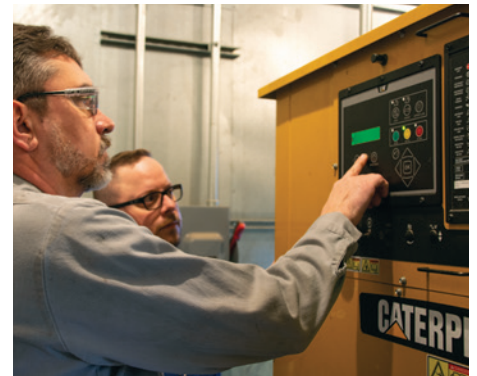
During the planning stage of the site upgrade, Andrew Watkins, manager of TierPoint's Lenexa data center, visited the Cat Switchgear facility as part of a factory witness test.
