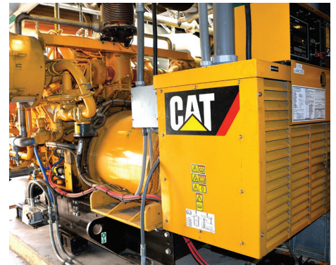
This Cat G3508 gas generator set has been supplying 50 percent of the treatment plant's power needs since 2005.
