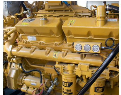
VCOM installed a Cat G3412 gas generator to back up the utility feed at the Auburn campus when the building first opened.
