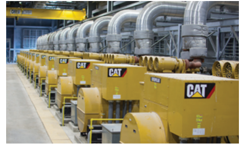
The 17th Street canal station is supported by Cat® diesel generator sets, switchgear and automatic transfer switches.
