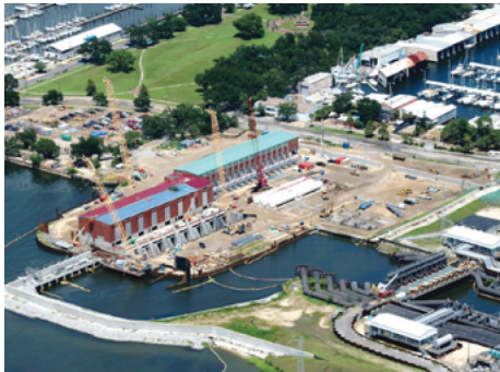
Three new pump stations protect the New Orleans area from devastating flood damage.
