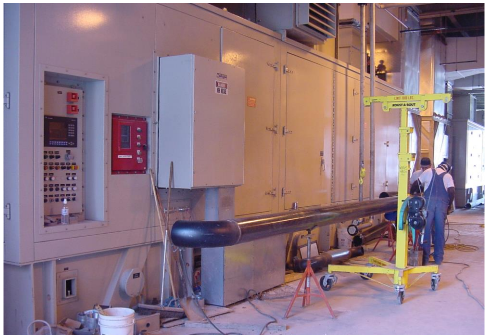
7.0 MW Solar Taurus Turbine Generator
