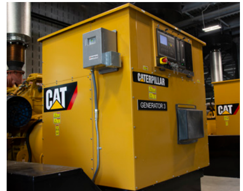
Michigan Cat supplied four Cat® C32 diesel generator sets that offer onboard paralleling through the Cat EMCP 4.4 control system.
