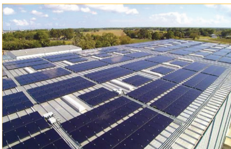
Louisiana Cat installed 1,550 Cat® PVT115 photovoltaic solar panels atop its service building.
