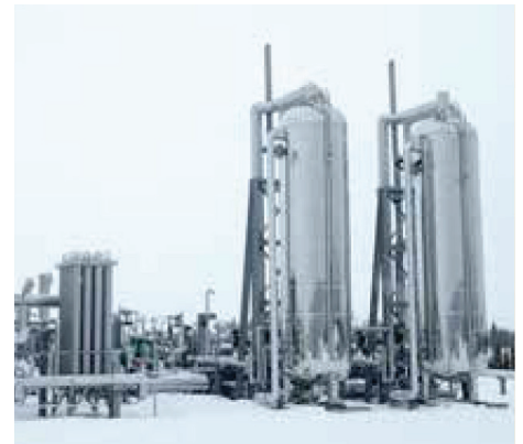
Renard mine, first gas power plant in Canada.
