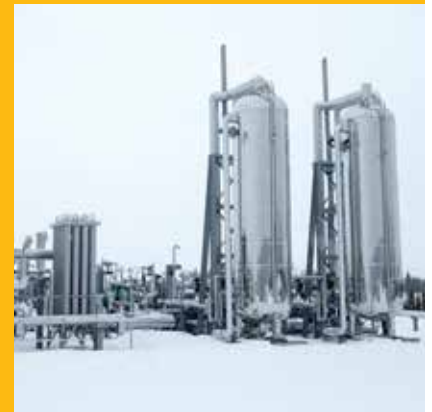
Renard mine, first gas power plant in Canada
