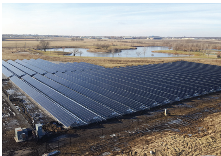
Built on an eight-and-a-half-acre site, the solar facility in Rantoul, Illinois, USA, repurposes an underutilized property at the former Chanute Air Force Base.
