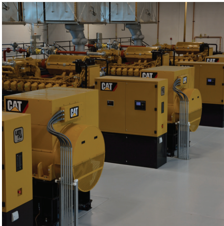
Powered by five Cat® G3520H generator sets, the Provo Power Plant is now considered the cleanest burning natural gas-fired power plant in the state.
