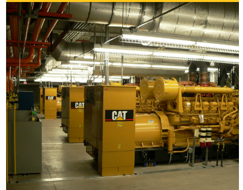
Four Cat® 3512B 1,500 kW generator sets provide reliable backup power to meet the requirements of this major university research hospital and regional medical center.
