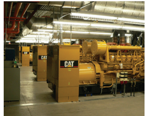
Four Cat® 3512B 1,500 kW generator sets provide reliable backup power to meet the requirements of this major university research hospital and regional medical center.
