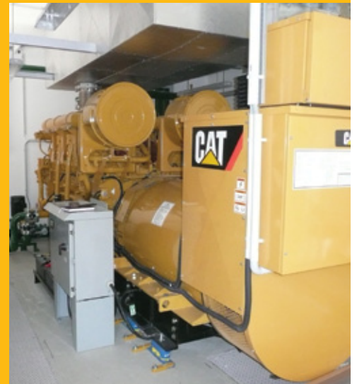
A Cat® 3516B-HD 2500 kVA diesel generator set supplies standby power for DoclerWeb's data center and other company facilities.
