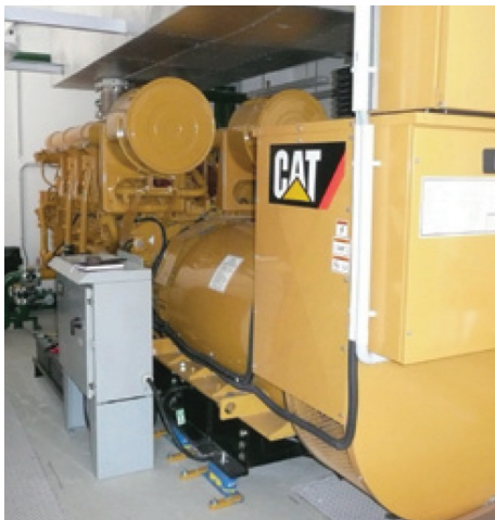
A Cat® 3516B-HD 2500 kVA diesel generator set supplies standby power for DoclerWeb's data center and other company facilities.
