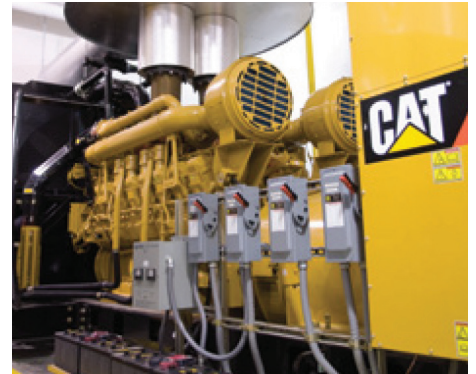
Four Cat® 3516C diesel generator sets produce 10 MW of power to provide essential emergency power needs for the Cape Fear Valley Medical Center's Valley Pavilion, Patient Services Tower and Central Energy Plant.
