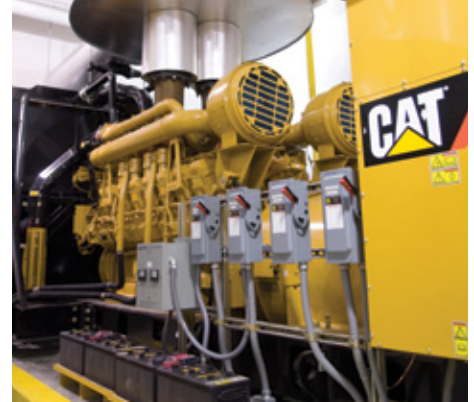
Four Cat® 3516C diesel generator sets produce 10 MW of power to provide essential emergency power needs for the Cape Fear Valley Medical Center's Valley Pavilion, Patient Services Tower and Central Energy Plant.
