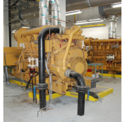
Cat diesel generator sets supplied reliable power continuously for 35 days after a 2010 fire at NCH's downtown Naples hospital.
