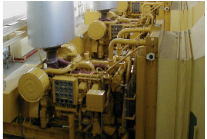
Three Cat 3508 generators provide 700 kW of standby power each to the St. Francis Hospital complex in Peoria, Ill.
