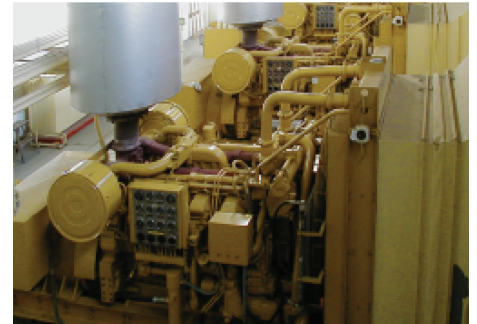
Three Cat® 3508 generators provide 700 kW of standby power each to the St. Francis Hospital complex in Peoria, IL.
