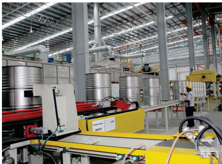
A Cat® generator set provides prime power for the facility's eight-hour shift, six days a week.
