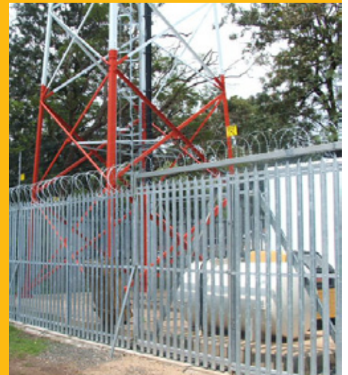
Alan Dick East Africa has used hundreds of Cat® and Olympian™ generator sets to supply power for cell sites.
