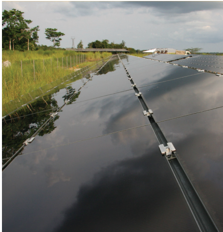
Local Cat® dealer, Tractafric Equipment, designed and installed a solar power plant consisting of 420 Cat PVT110 solar panels.
