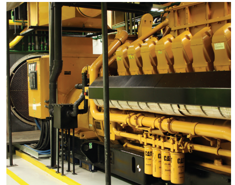
Four Cat G3520C generator sets generate electrical energy—up to 8 MW—capable of meeting a constant 100 percent load for the Rochaverá Corporate Towers complex.
