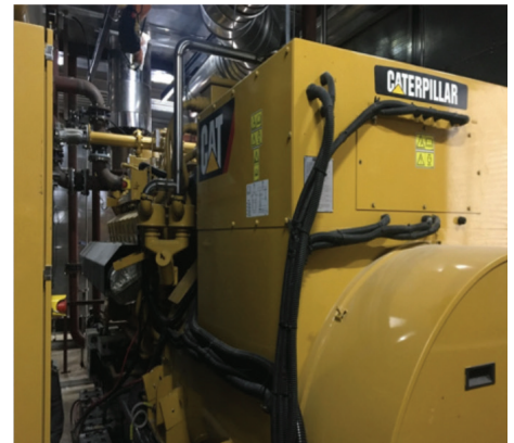
For Phase 1, two Cat® G3520H gas engine generator sets with a full load rating of 2,500 kW were installed.
