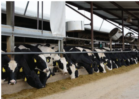
Homestead Dairy installed a biomass waste-to-energy facility, including two anaerobic digesters, to process the manure from more than 2,000 cows.
