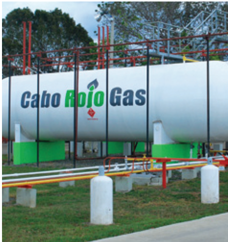
Cabo Rojo Gas requires reliable, efficient standby power at their five distribution centers to keep pumps working and their delivery trucks on the road.
