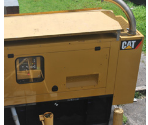
An Olympian™ 100 kW D100-6S diesel generator set was installed in 2010, which provides backup for the entire bakery including the air conditioner, lighting, coolers, ovens and cash registers.
