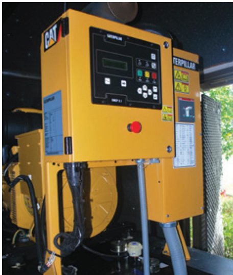
Interlink builds engine rooms with sound-attenuating padding at the back of the residences to ensure the quietest operation possible.
