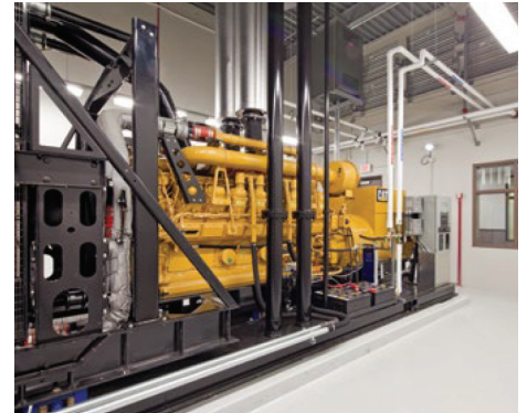
NMC Power Systems installed four Cat® 3516 diesel generator sets and a customized Cat switchgear system to power Scott Data Center, earning the building a Tier 3 certification.
