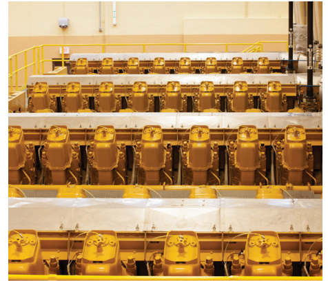
Four Cat® G16CM34 gas generator sets produce 25 MW of power to supplement power generated from wind sources.
