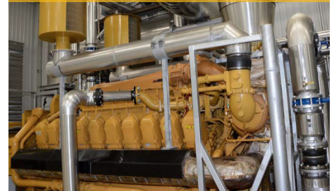
Toromont Power Systems installed two high-efficiency Cat® G3520C natural gas generator sets providing 4 MW of power to anchor the CHP system.
