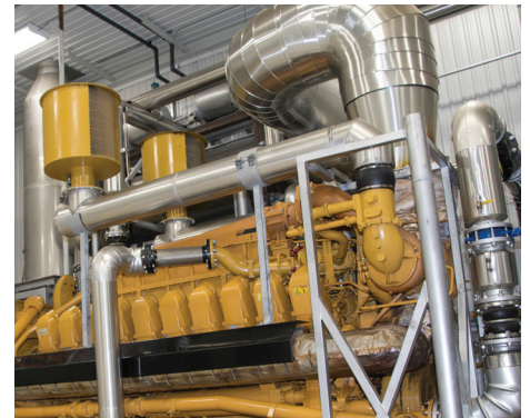
Toromont Power Systems installed two high-efficiency Cat® G3520C natural gas generator sets providing 4 MW of power to anchor the CHP system.
