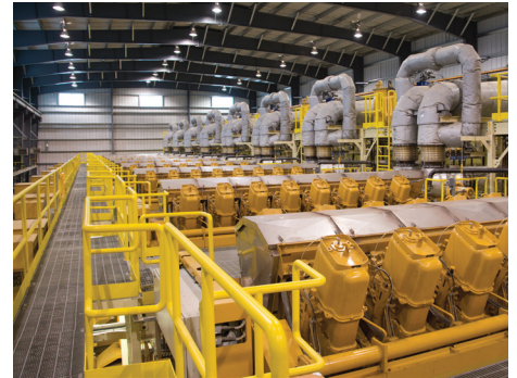
ANC commissioned an on-site 65 MW natural-gas-fired power plant with 10 Cat® G16CM34 generator sets.
