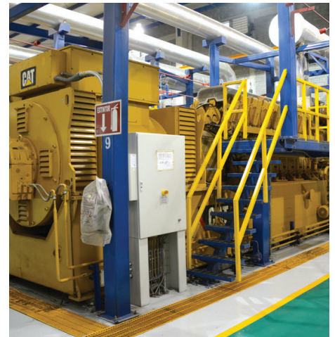
40 Cat® CG260-16 generator sets produce 160 MW of power for four separate plants at AHMSA.
