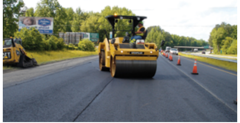
There are no drum stop marks in the fresh mat when the compactor is able to roll onto a cold, compacted mat.
