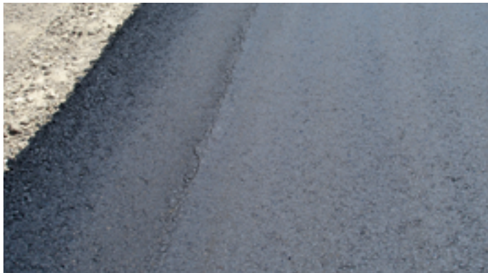
Crack in the mat along drum edge set back from the unconfined edge.
