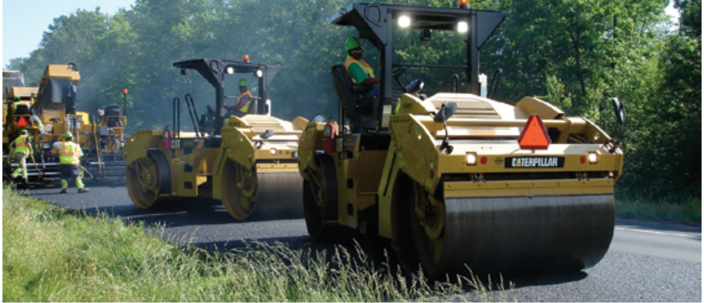
Two initial phase compactors reversing direction behind a paver. Note angled stop.
