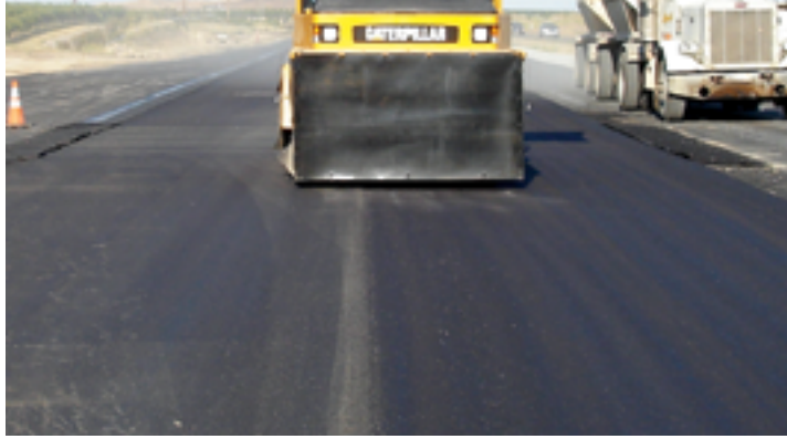
Pneumatic compactors in the intermediate phase are effective at sealing hot / cold longitudinal joints.
