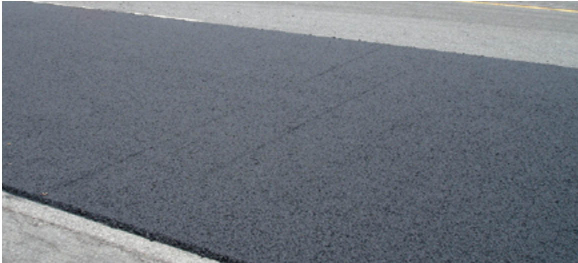
Screed imprint in the bituminous layer created by stopping the paver.
