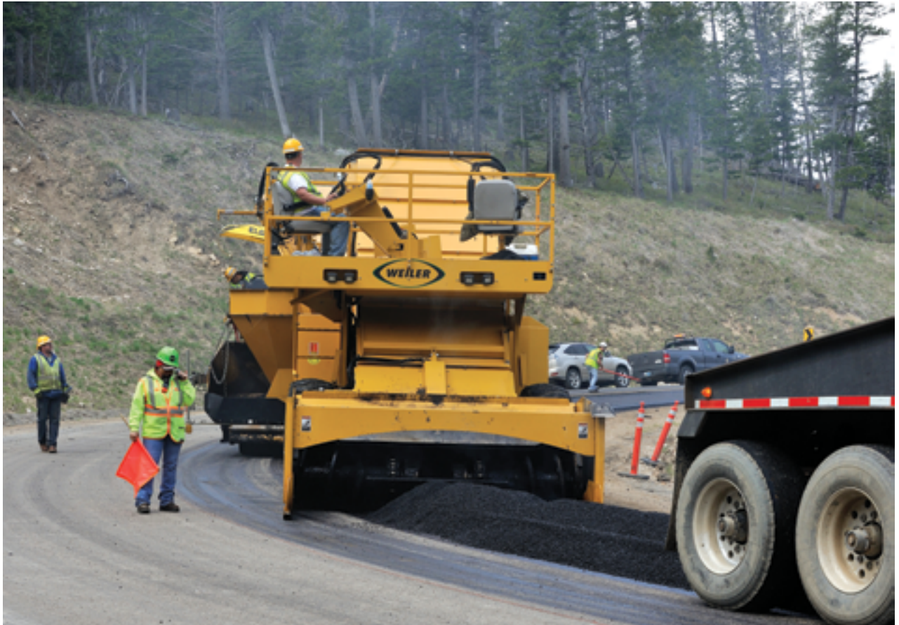
Material transfer devices, this one equipped with a windrow elevating head, enable the paver to operate continuously at the same speed.
