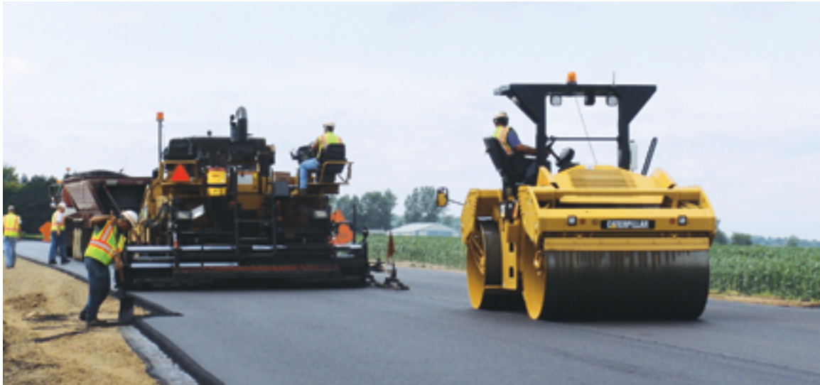
Sealing the longitudinal joint during the first pass improves the appearance of the joint.
